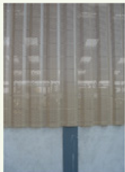
Bardage bac acier perforé
